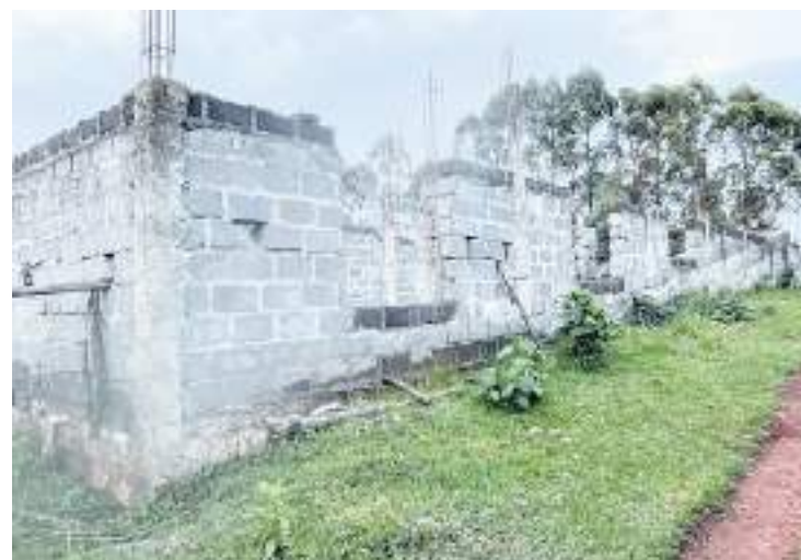
The stalled community library project in Nandi county /MATHEWS NDANYI
