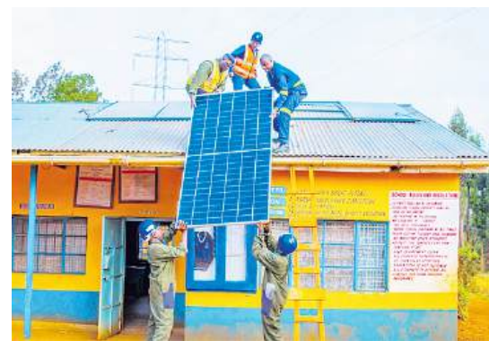
Workers instal solar panels at Riabai Primary School in Kiambu Town constituency /ALICE WAITHERA
