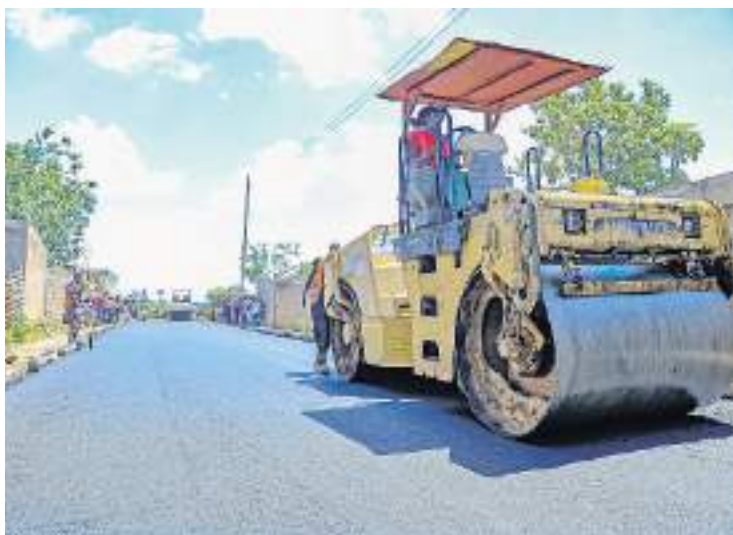
A contractor works on one of the road projects funded by the World Bank in Eldoret City /MATHEWS NDANYI
