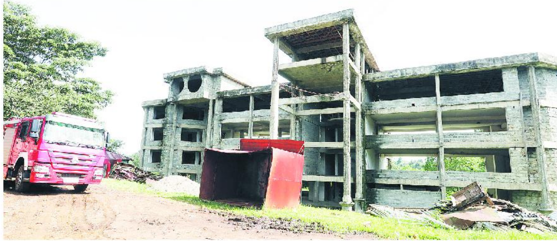
The Sh150 million Nandi County Government offices in Kapsabet. The construction has stalled for over seven years now. [Kevine Tunoi, Standard]
