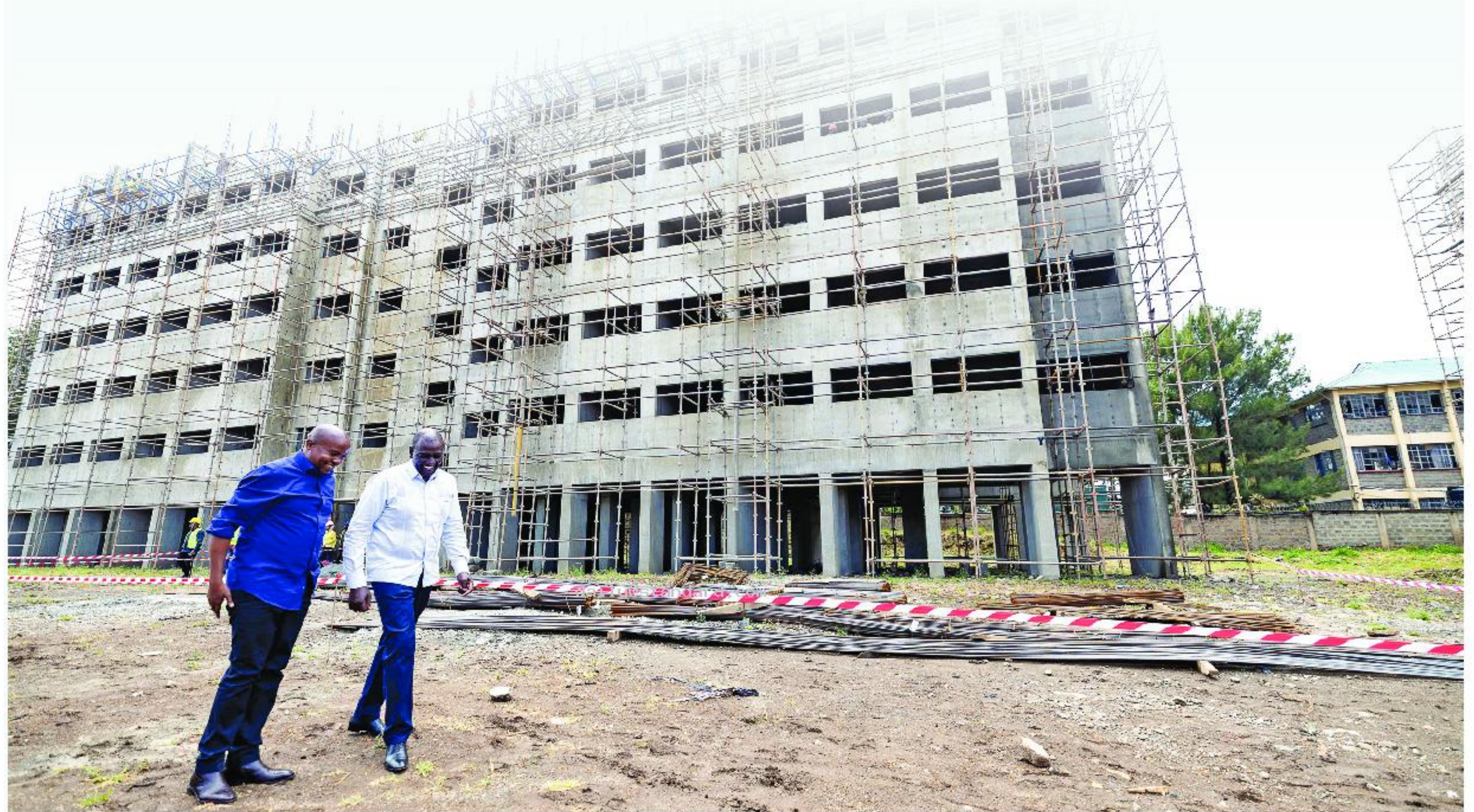
President William Ruto and Deputy President Prof Kithure Kindiki inspect the ongoing construction of the 4,566-unit Shauri Moyo B Affordable Housing Project in Kamukunji Constituency, Nairobi, earlier this year. [PCS]
