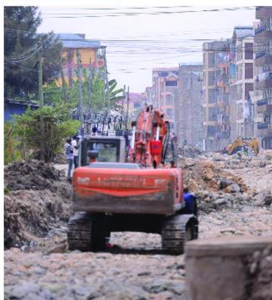
Roadworks are currently ongoing on SDA Road in Umoja 1 Ward, Embakasi West. [Courtesy]
