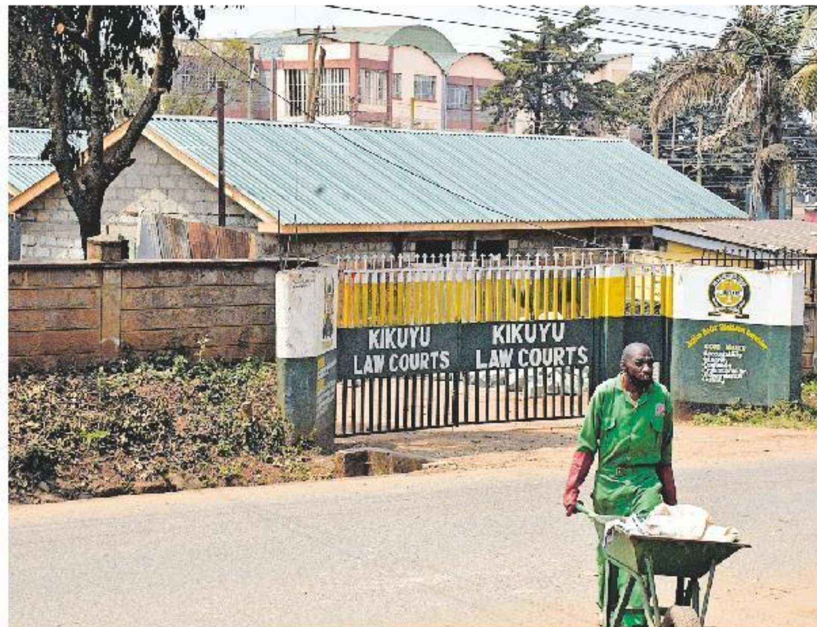
Kikuyu Law Courts in Kikuyu town, Kiambu County, under construction on Thursday. The court was set ablaze during the June 25 Gen Z protest anniversary. FRANCIS NDERITU / NATION
