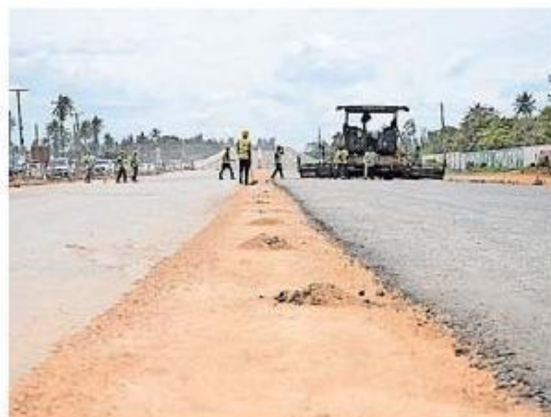
Ongoing construction of the Mombasa-Mtwapa highway on Thursday last week. WACHIRA MWANGI | NATION
