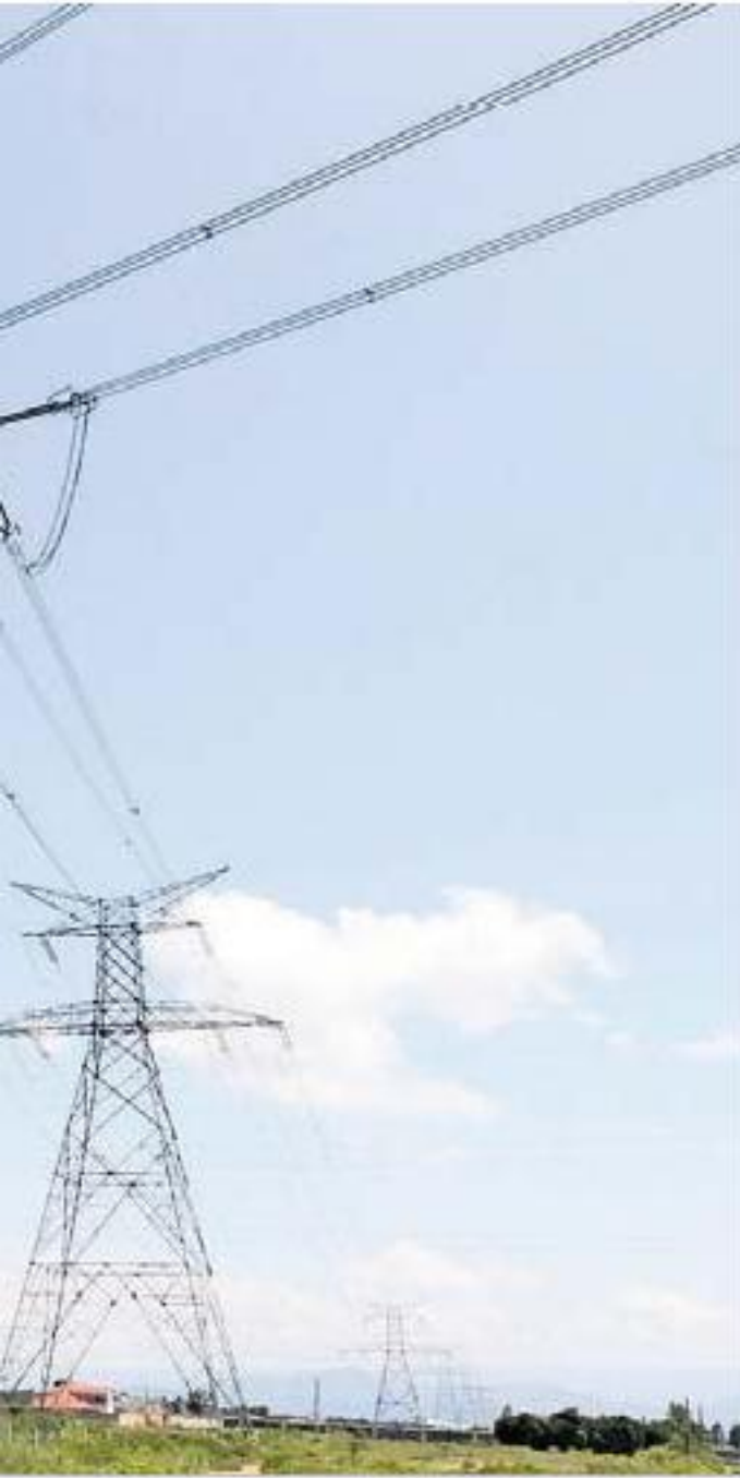
A power transmission line in Lon-gonot, Nakuru County, on May 15. Ketraco faces a Sh8.7 billion bill for the termination of a contract awarded to a Spanish firm for construction of the Lessos-Tororo transmission line. BONIFACE MWANGI | NATION
