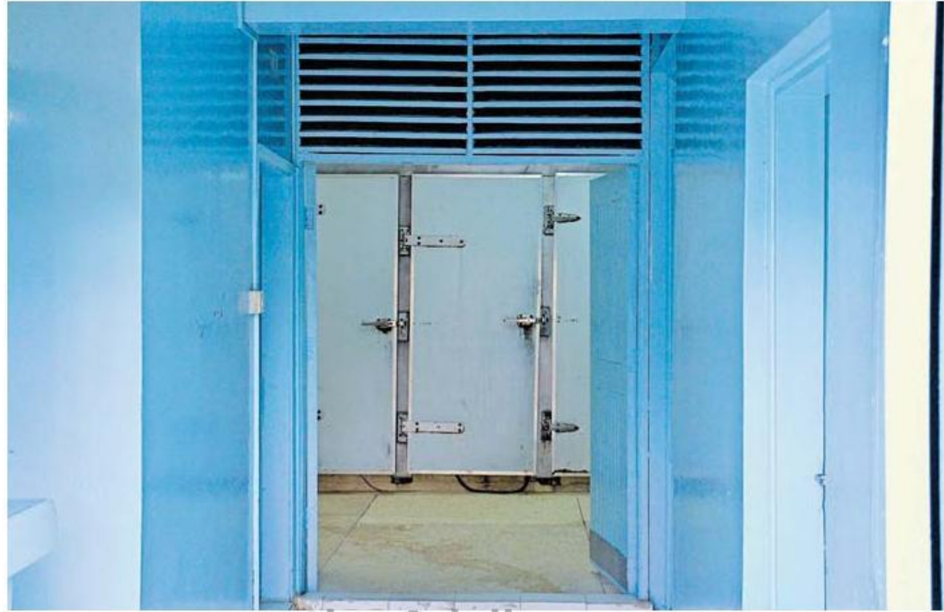
The freezers used to store bodies at Nairobi Funeral Home.
