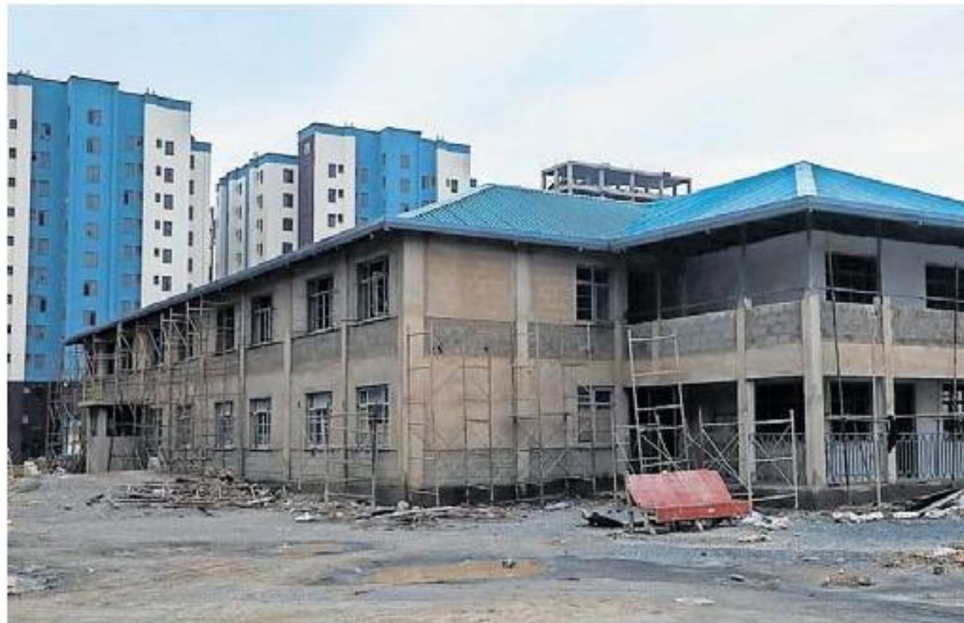
Ongoing construction of the Mukuru Phase One School in Nairobi. In the background is the New Mukuru Housing Estate Phase One, whose beneficiaries moved in, in May.
