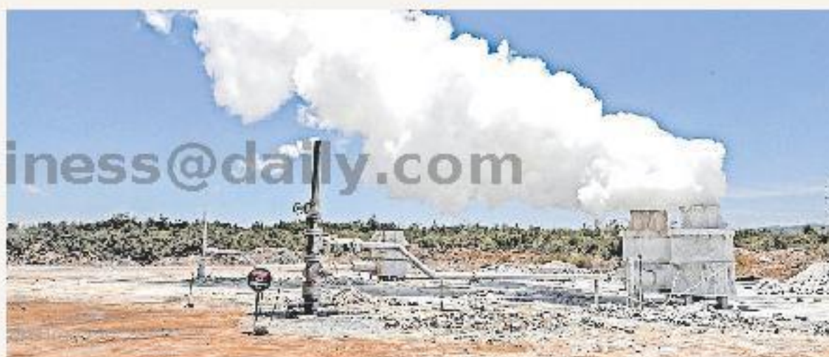
A geothermal well in Olkaria, Naivasha, on February 21. DENNIS ONSONGO
