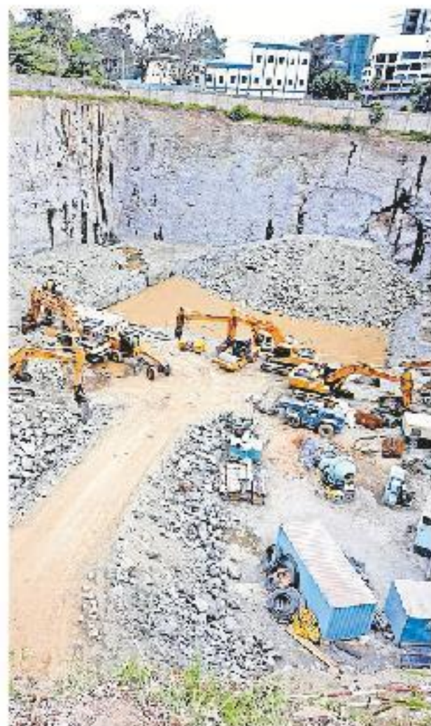
Equipment at the construction site of the proposed Africa's tallest building in May, 2017. Credit bank can now auction
