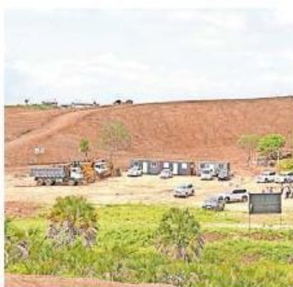
The Taifa Gas plant construction site in Dongo Kundu, Mombasa. WACHIRA MWANGI
