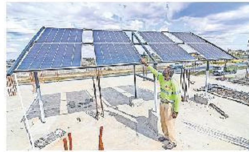
Fredrick Omondi, co-founder of Kimalat Holdings, stands next to solar panels at the farm.
